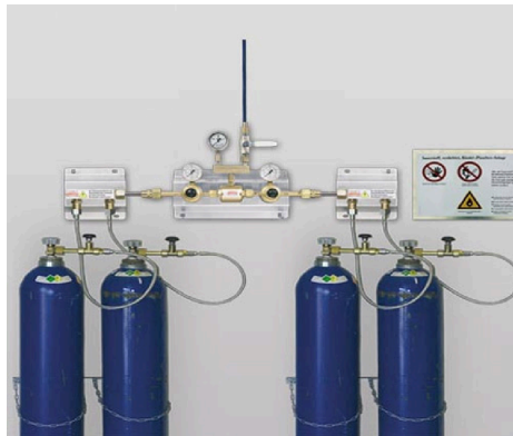
Figure 19: Gas Cylinder Manifold
